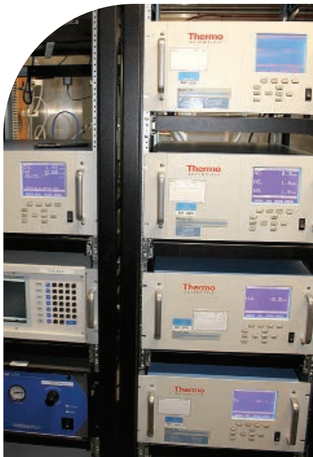
Figure 2: Interior photo of the KPP Station
