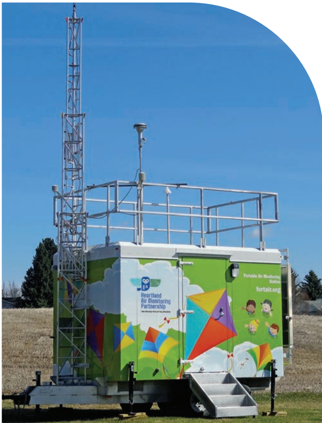
Figure 1: Exterior Photo of the KPP Station
