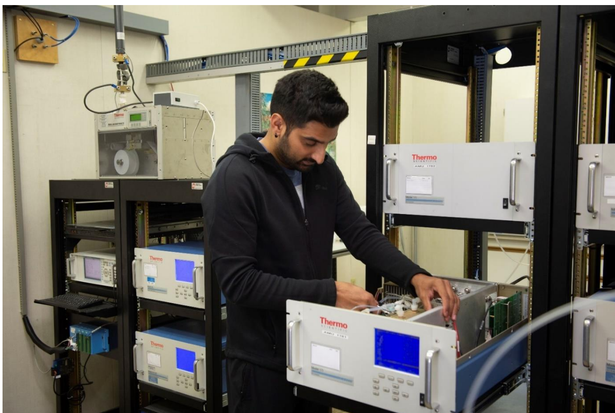
Figure 2: Continuous air monitoring station interior
