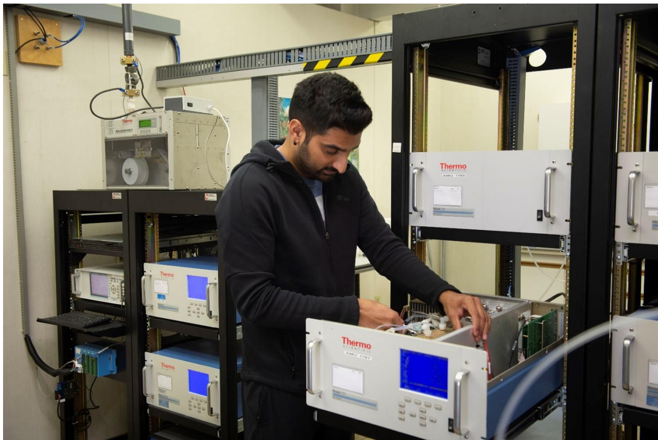
Figure 2: Continuous air monitoring station interior
