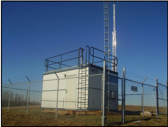
Figure 7: Lamont County Station
