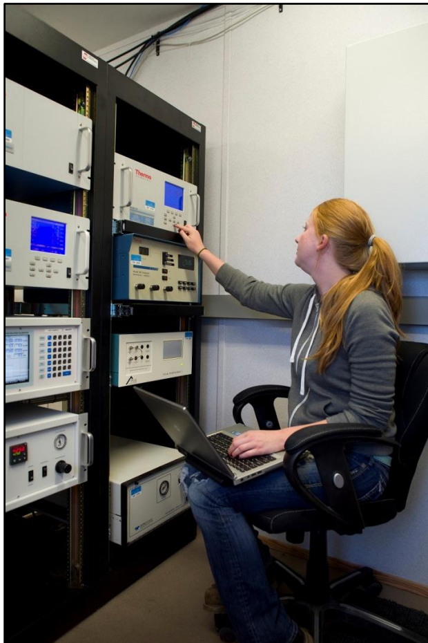
Figure 1: Continuous air monitoring station
