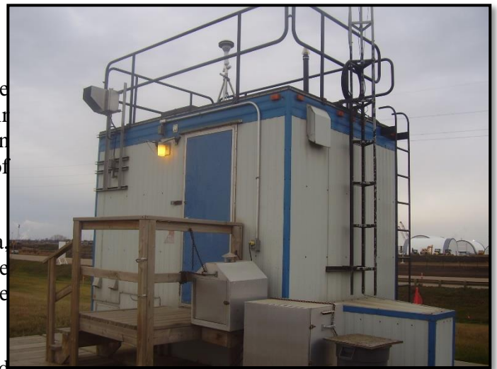
Figure 9: Redwater Industrial Station
